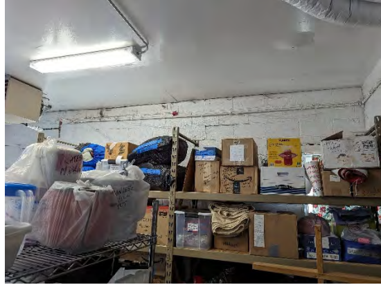
Photo 6: CMU horizontal cracking
