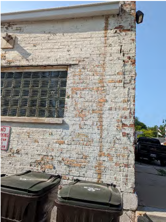
Photo 3: NW corner cracking
