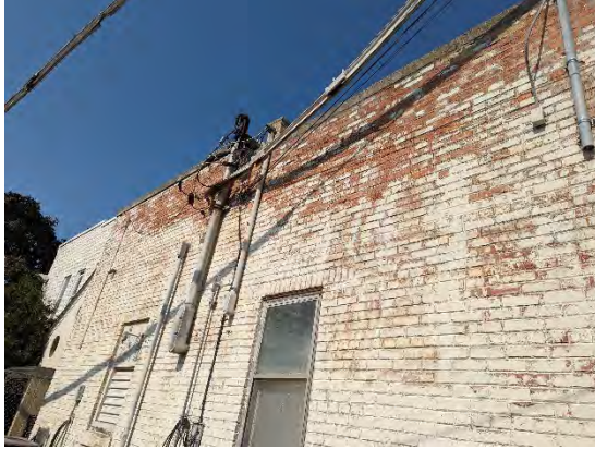
Photo 1: Spalled brick on East elevation
